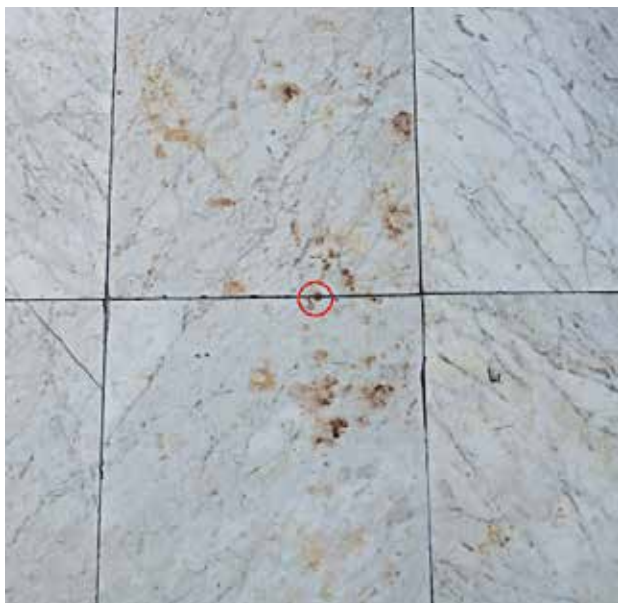
Figure 1. Stains from the floor in the staircase of the Staszic Palace. Test stain marked with a red circle
